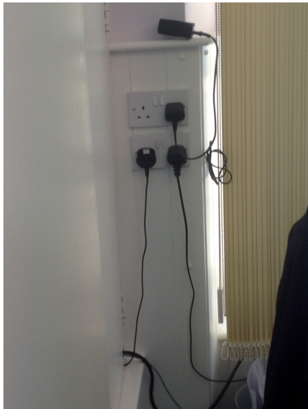
Figure 15: Raised wall sockets for safety.
