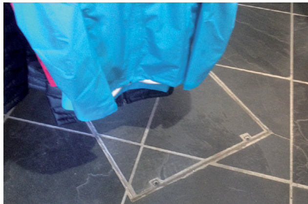
Figure 12: Firm fixing of an under floor drain that previously caused internal flooding.
